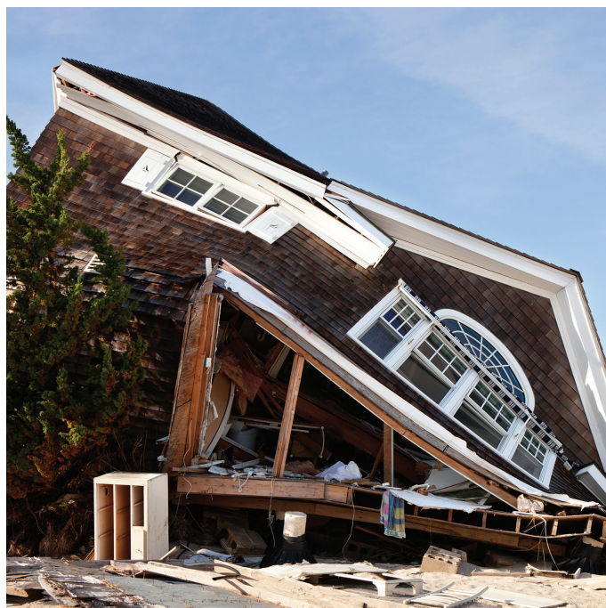
Storm-damaged home after Hurricane Sandy.
